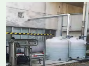
Greywater storage tanks
